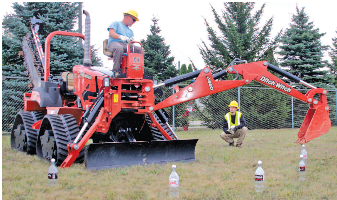
Great Lakes Energy lineworkers practice their digging skills in a timed exercise that involves knocking off the golf balls without knocking down the bottles, too. Part of their work includes installing underground power lines which requires knowing how to safely operate the necessary equipment. Other training exercises for lineworkers were held, too, as part of field training day held recently at their Boyne City headquarters.
